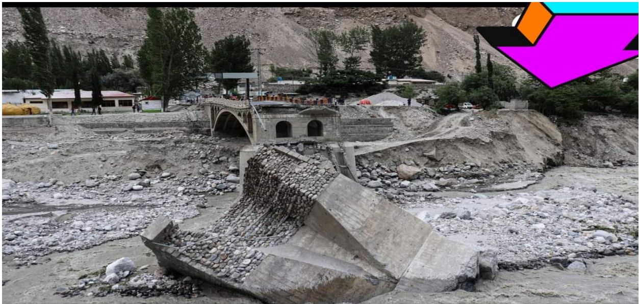
FIGURE 15: DAMAGE OF HASSANABAD BRIDGE (7 MAY 2022)
