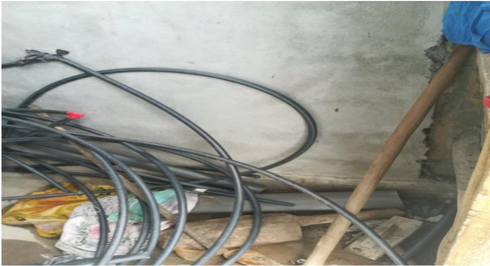
Figure :1 Washroom of Tmeer e Public school Ali sojal
